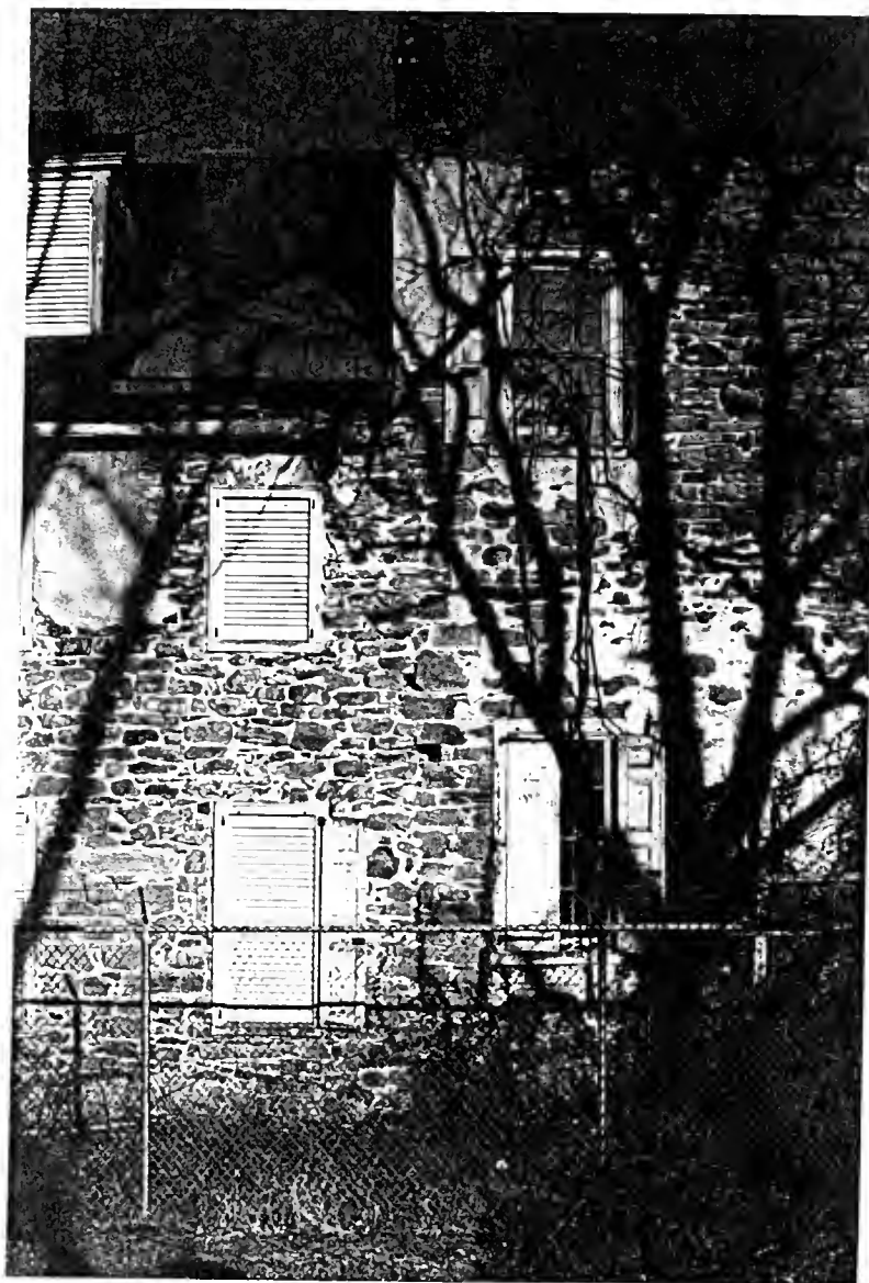
Figure 13: Connection along west wall between the Pawling section (to the left), and the Wetherill addition. Notice the height differential between the two sections and the continuous partition wall which separates them.
